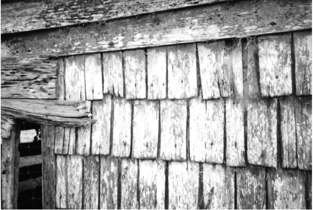
Figure 5.13. Wooden shakes or shingles cover a portion of the north exterior of Room 1.
