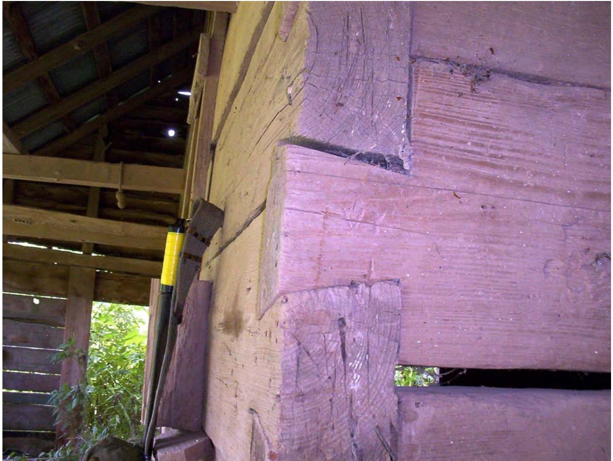
Figure 5.3. The carpenter's mark "VI" is visible on the end of this timber. This mark was used to insure easy assembly after notching the timbers.
