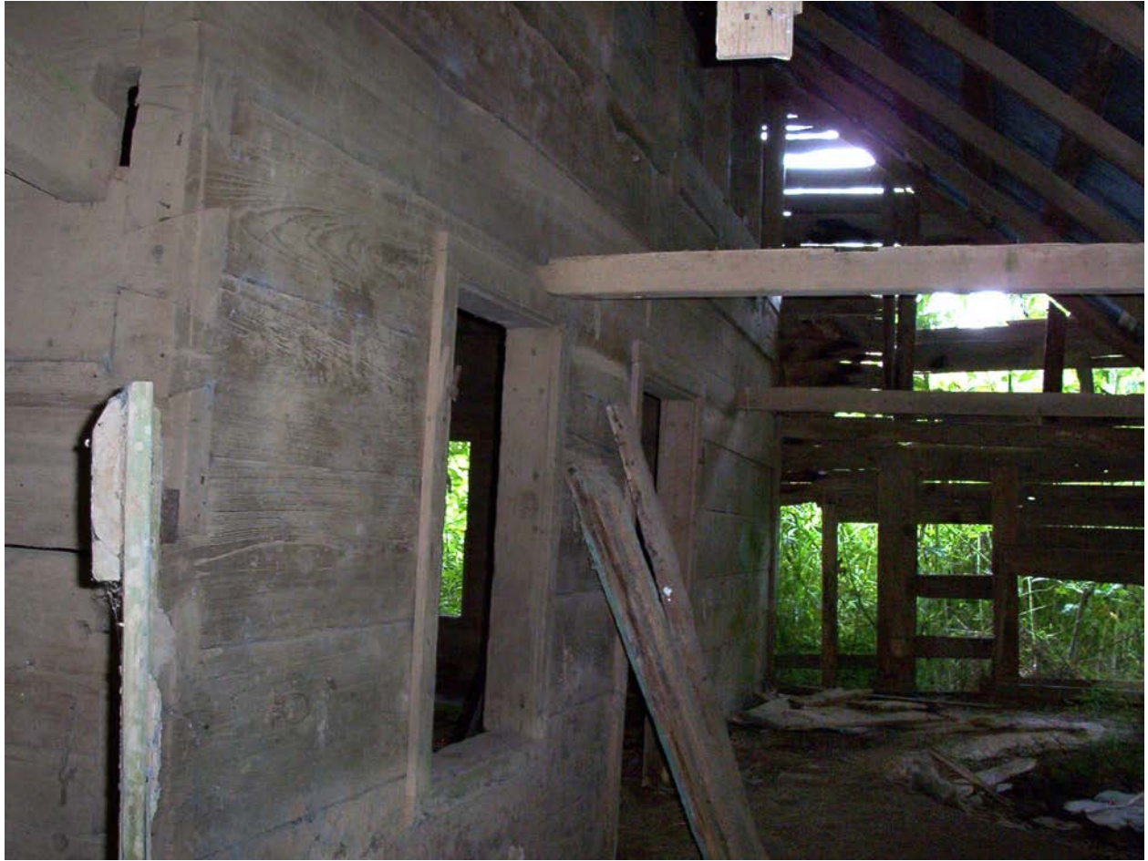
Figure 5.21. Ceiling joists were added during the Phase III construction of the “barn.”
