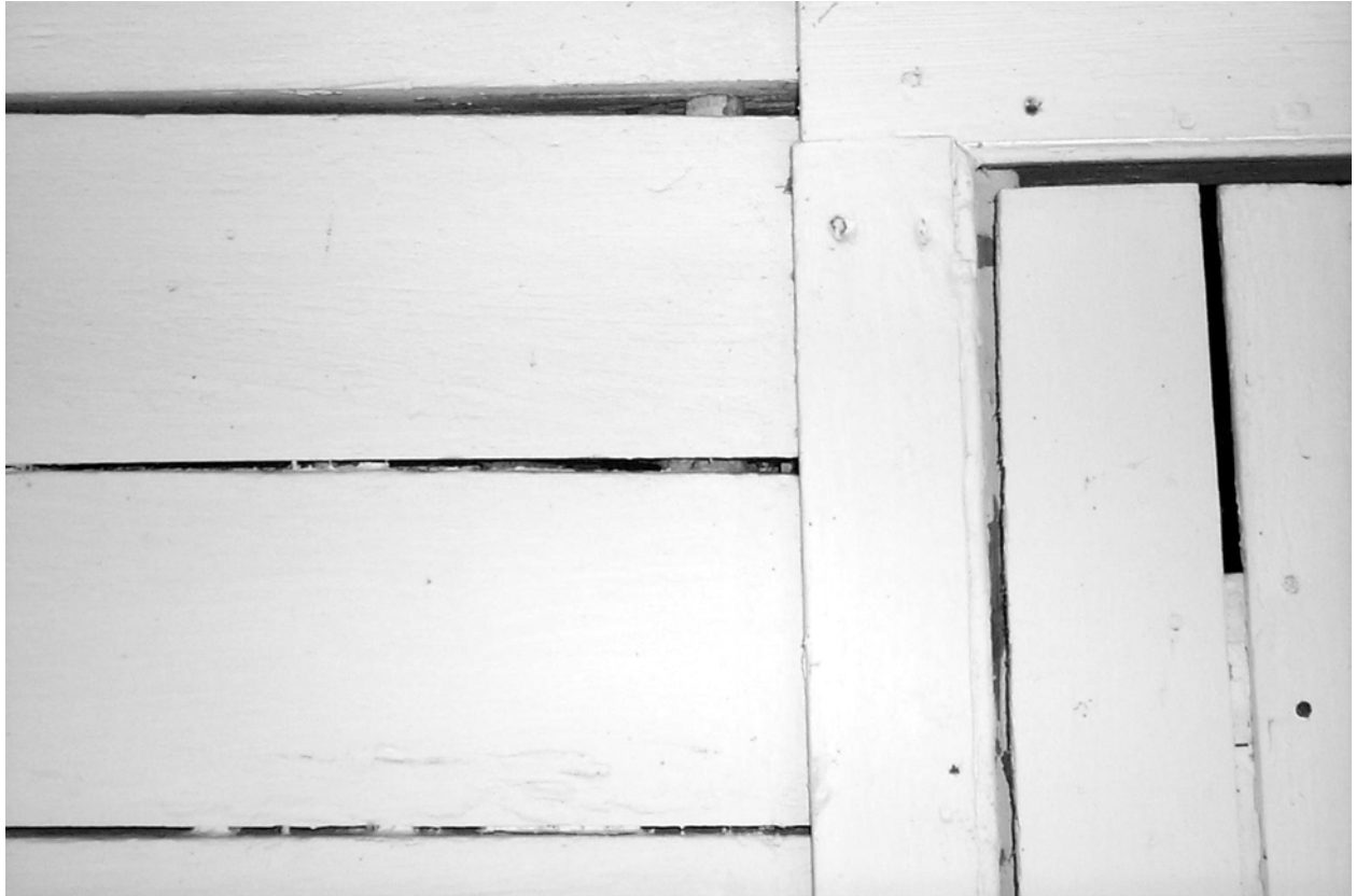
Figure 5.34. The timbers of the Rosedown Milk House are pegged above and below for more stability around the door and window openings. The pegs are visible above and below the second timber shown in the photograph.
