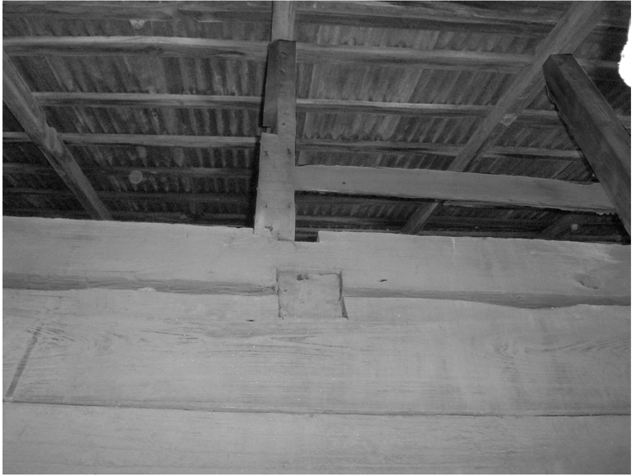
Figure 5.6. Ceiling joists are mortised through the two topmost timbers of the west and east walls of Room 1. Notches from the original roof joists are still visible (above the ceiling joist) and were partially reused for the uprights used to support the new roof. These uprights were created from used timbers, possibly from the original roof structure.
