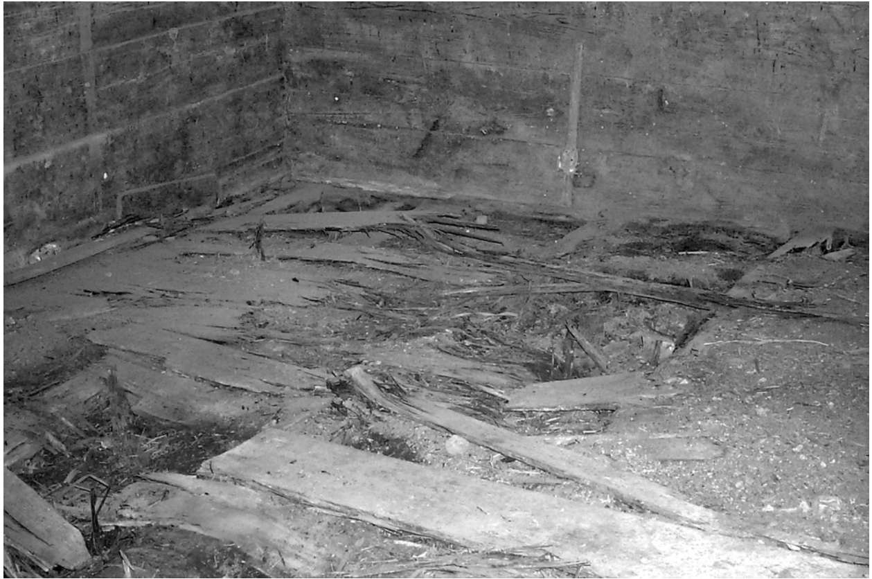
Figure 5.7. The tongue-and-groove floor is nailed to the floor joists and sills of Room 1.
