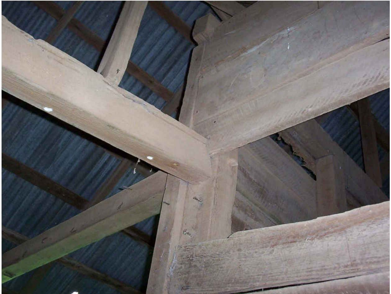
Figure 5.25. The same joist depicted in Figure 5.24 connects to Room 2 of the structure shown here.
