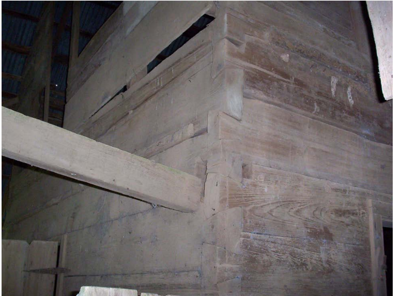
Figure 5.24. Joists were added between the two rooms of the “barn” to join the two ceilings and further stabilize the building. The joist shown here has slipped out of its hole because the northern room has shifted.
