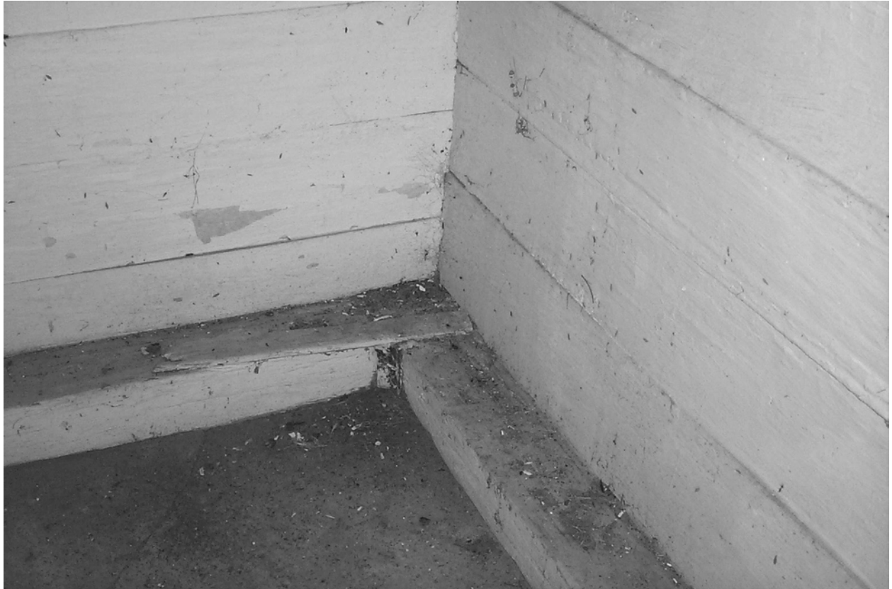
Figure 5.35. The sills of the Rosedown Milk House extend out into the structure. A floor was probably attached to the sill at one time.
