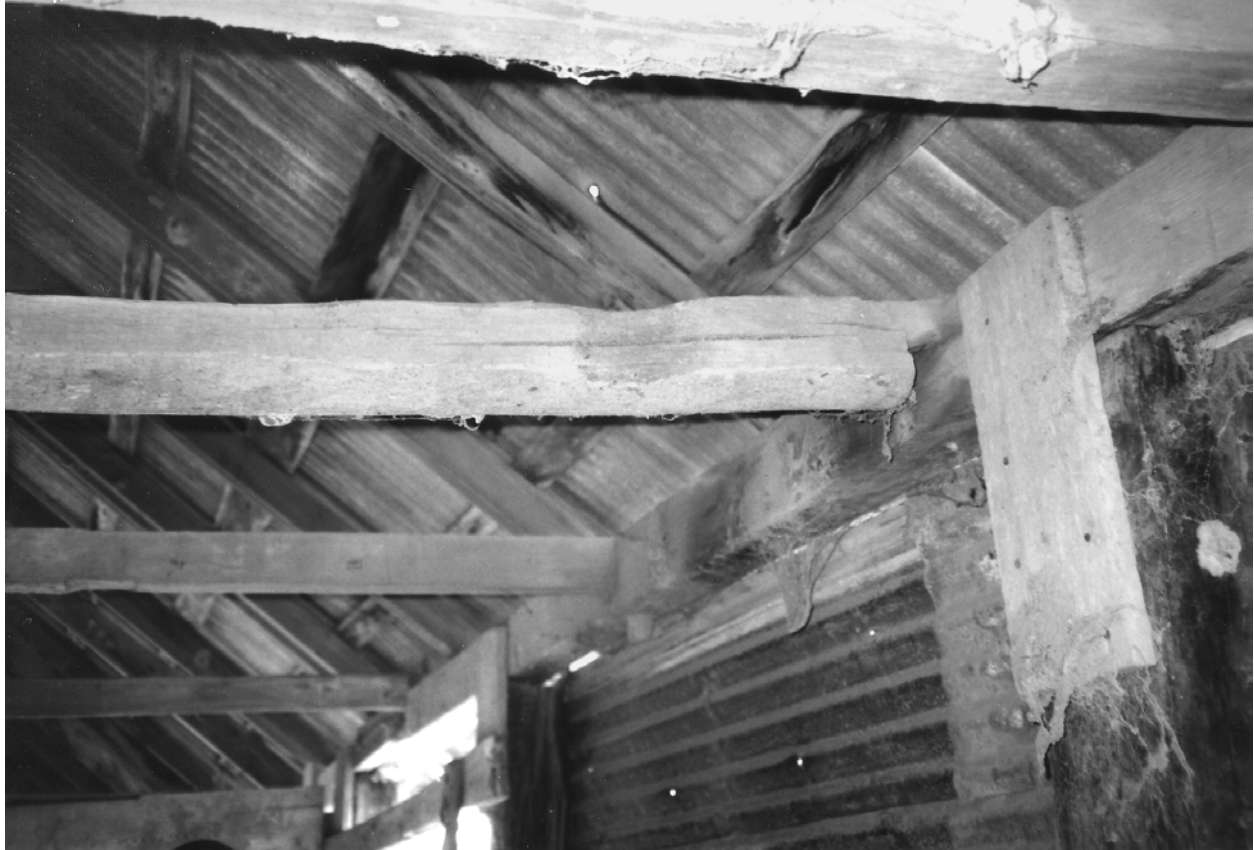
Figure 5.23. Some of the ceiling/roof joists were reused from another structure (see joist in background) and others were made with whatever was available. Note the tree in the foreground of the photograph that has been planed on two sides, but the bark remains on the bottom.
