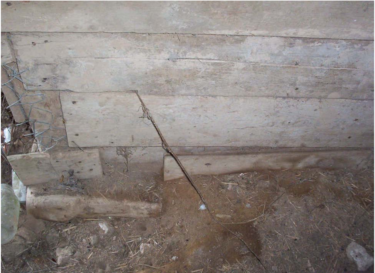
Figure 5.16. Room 2 rests on wooden piers shown in the lower left-hand corner of this photograph.
