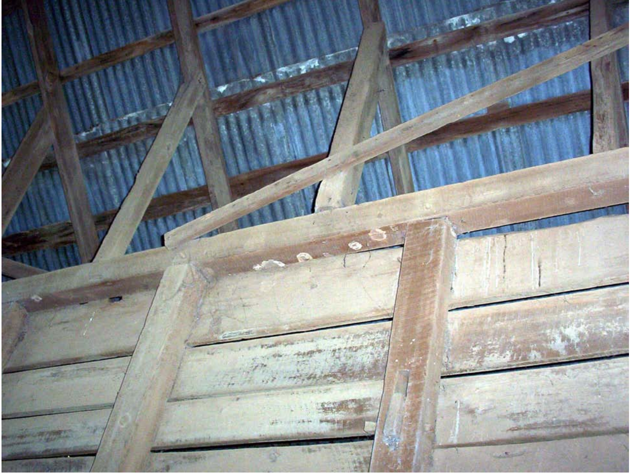
Figure 5.15. The same posts of Figure 5.14 are also mortised into a top plate.
